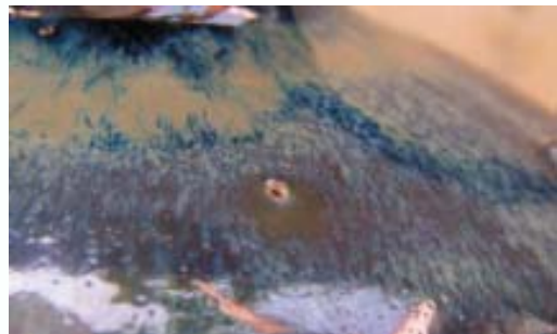
Pitting and blister
